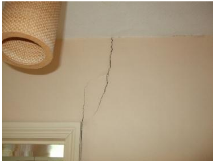
FIGURE 03 Landing - tapering crack above rear door
