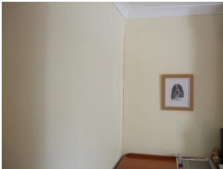
FIGURE 05 Rear bedroom - vertical crack at wall junctions.
