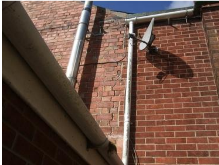
FIGURE 06 Rear elevation - vertical stepped crack
