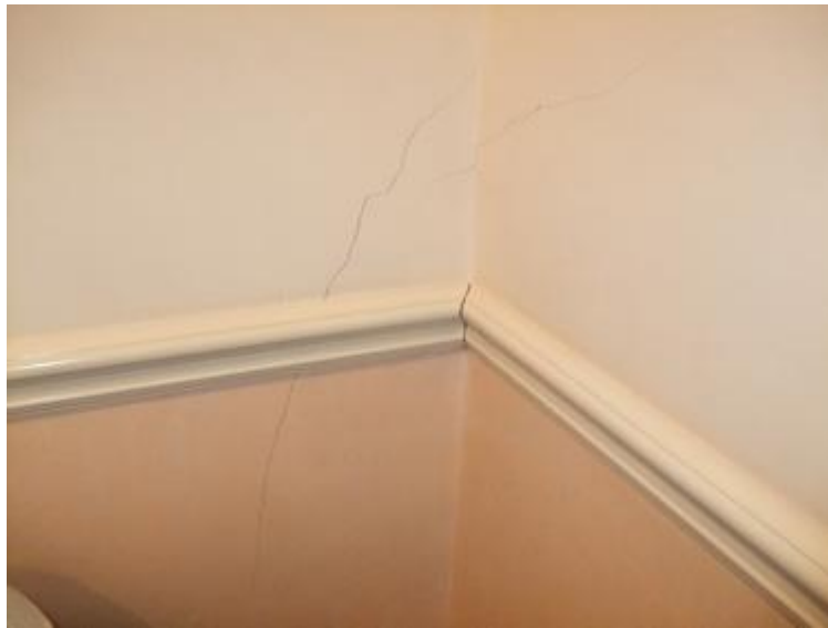
FIGURE 04 Hallway - crack to internal lounge wall
