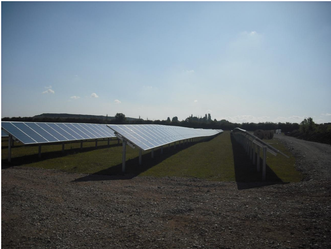
Similar but larger PV array
