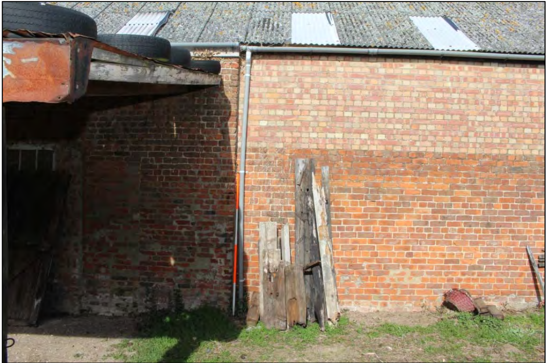
Photo 4: Overview of southern elevation showing butt joint between phases of extension/repair
