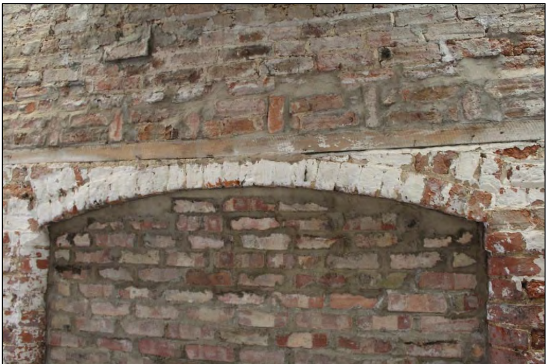
Photo 10: Detail of blocked up slots that may once have supported timber joists. Note the extant timber immediately below
