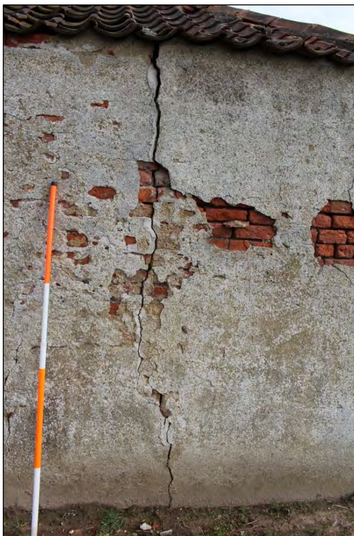
Photo 26: Evidence of cracking and erosion beneath cement render
