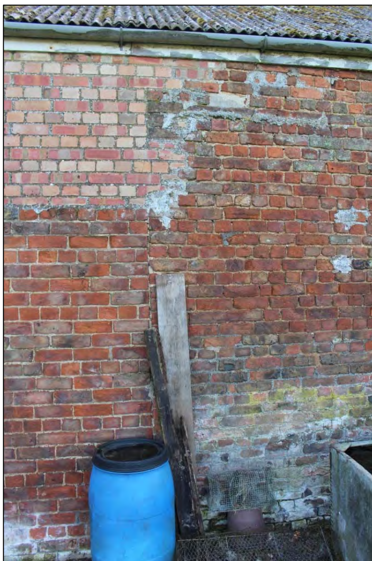
Photo 6: Detail of butt joint on northern elevation. Note the later brickwork to the upper courses, contemporary with the later extension
