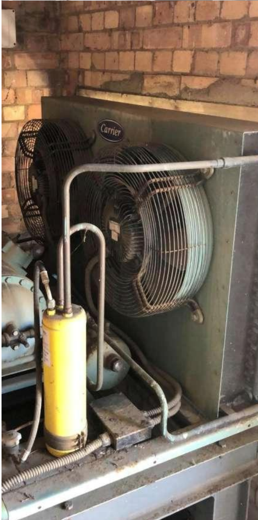
Photo 14 Refrigeration unit in small extension
