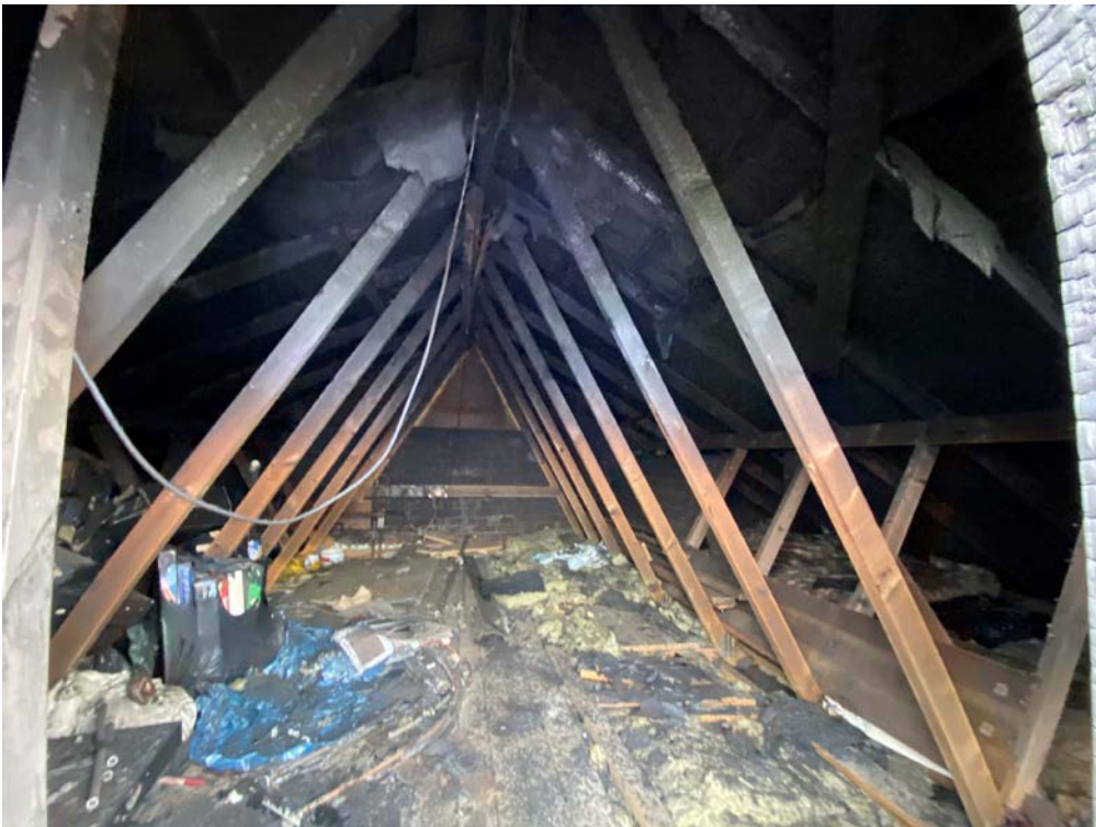
Photo 8 – Truss roof above kitchen extension appears to be in a reasonable condition but further inspection require upon removal of covering.
