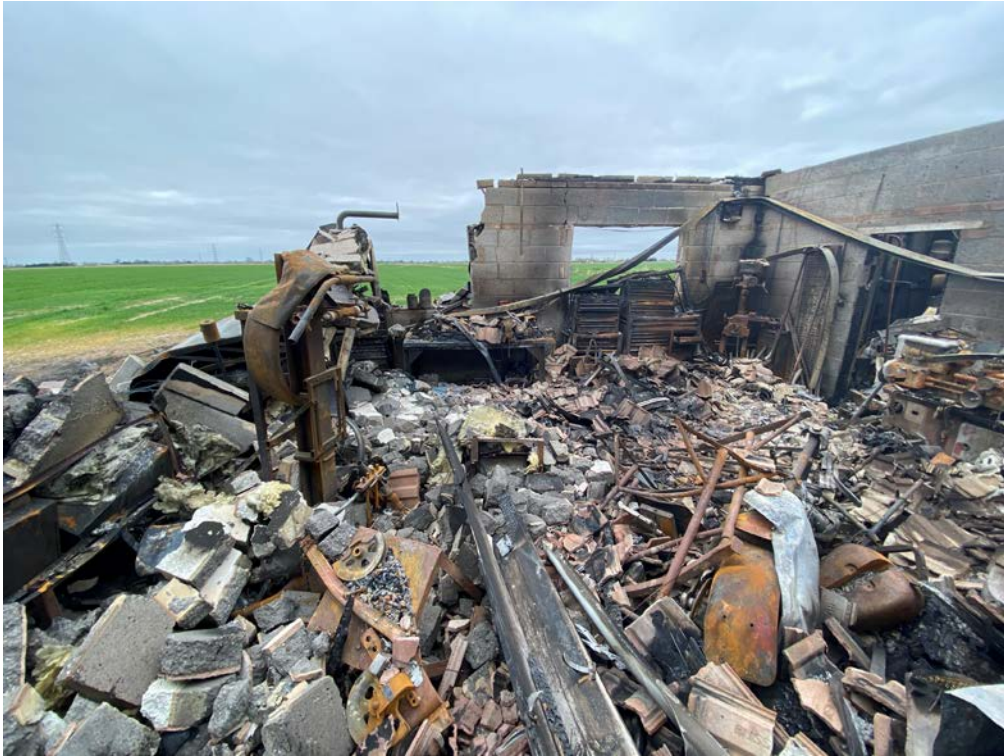
Photo 5 – Building F with failed left elevation, roof and covered in fire debris and contents.
