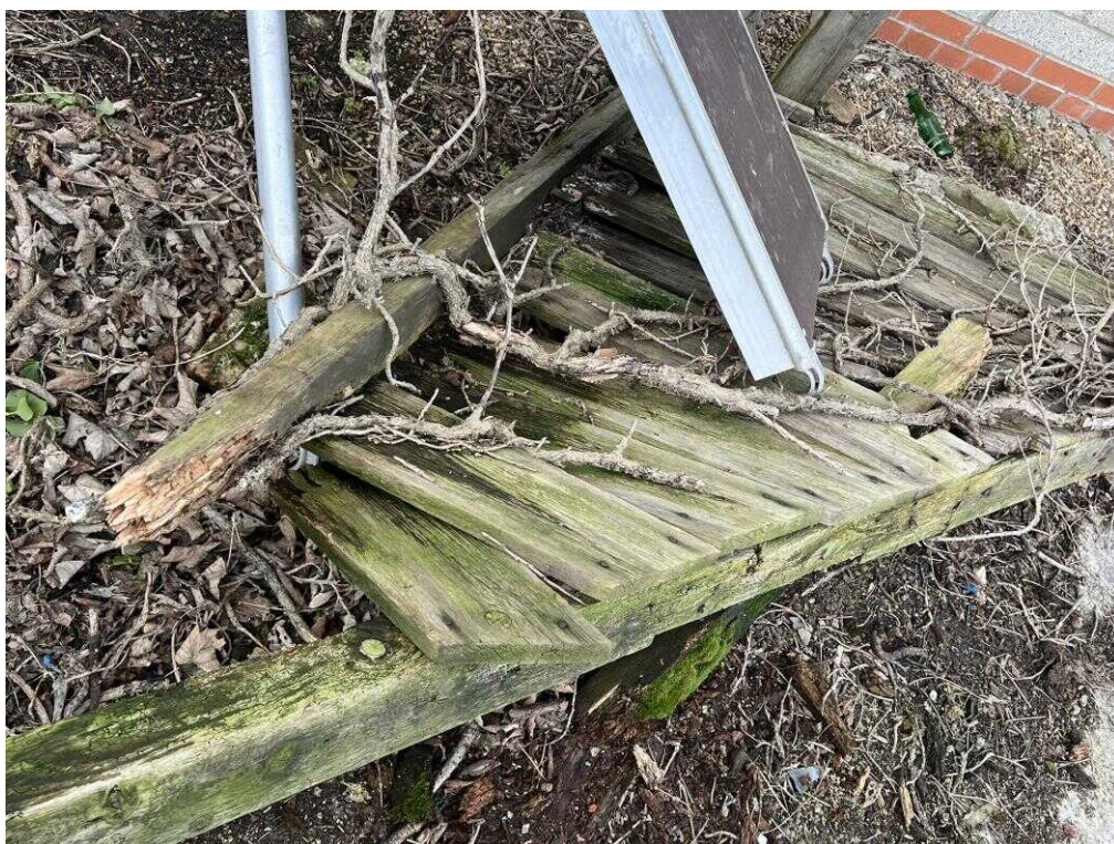
Fig. 32 – Collapsed weather-boarding infill from east gable of roofed-in area.
