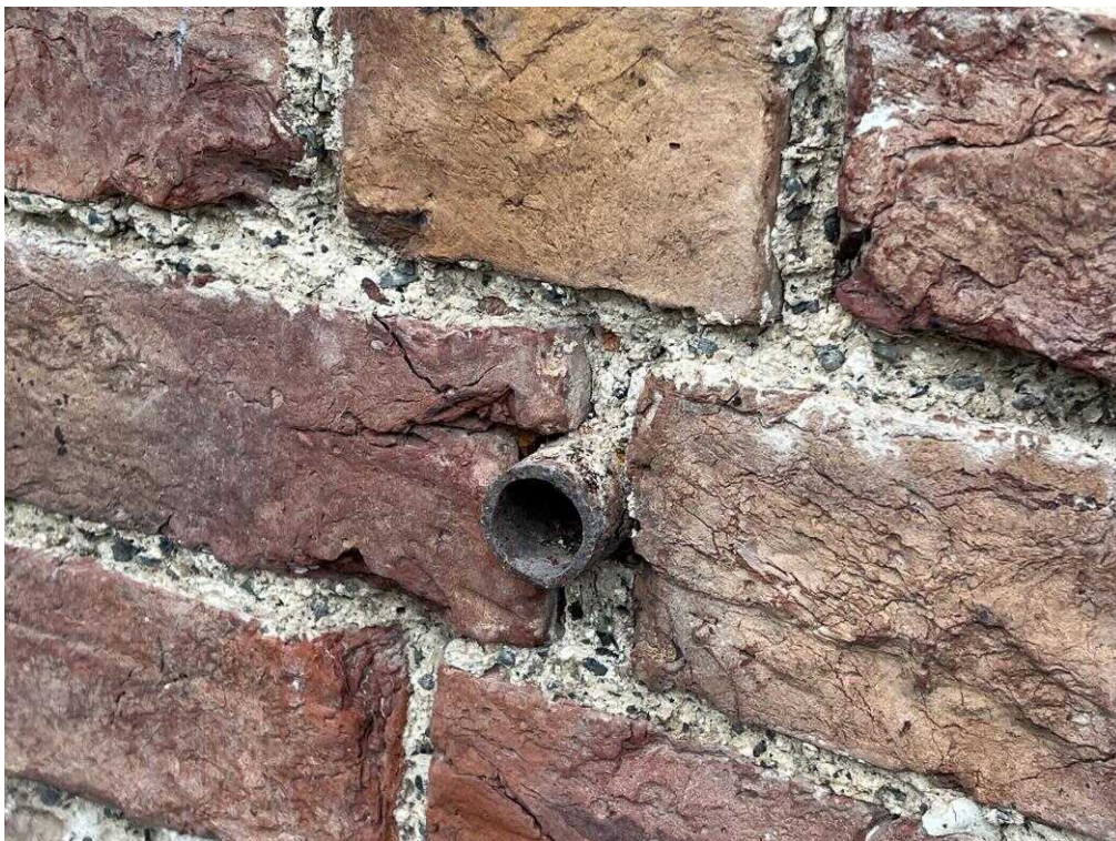
Fig. 42 – Redundant pipe through external wall.
