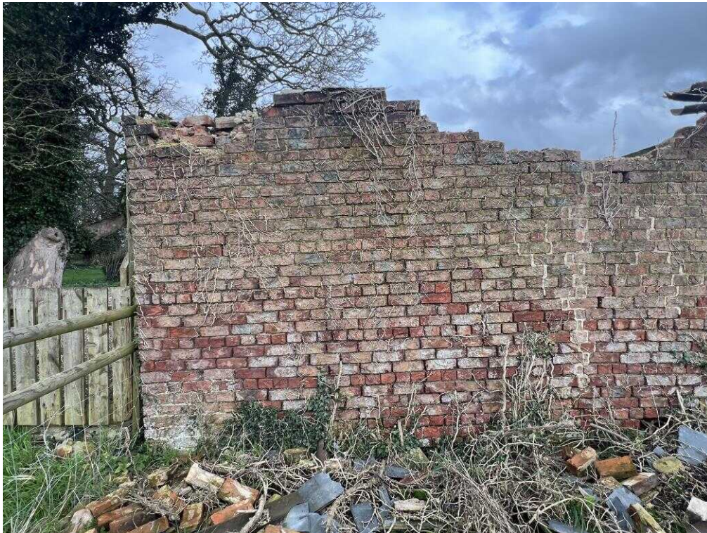
Fig. 21 – North section of west elevation with repaired crack in brickwork evident.
