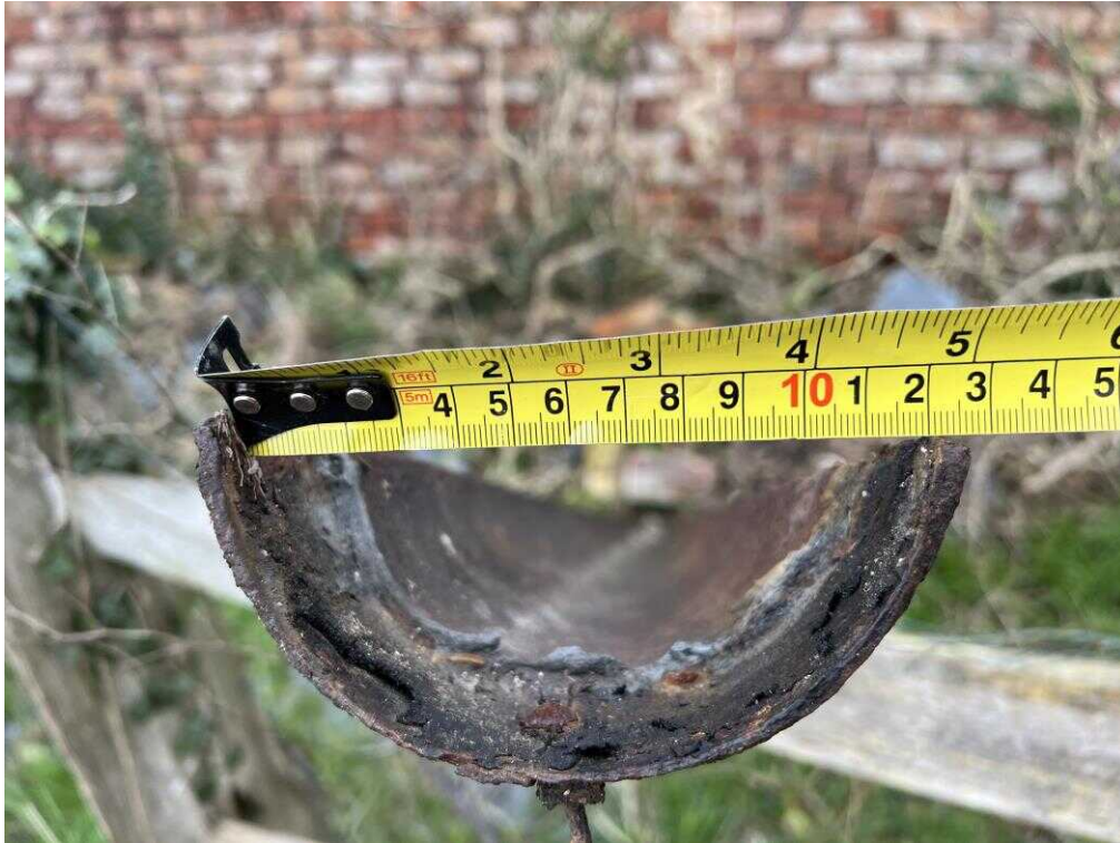
Fig. 27 – Cast iron half-round gutter section detail (loose on floor)
