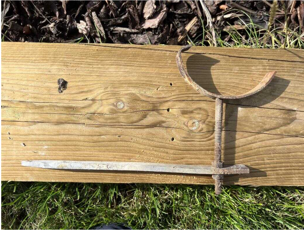
Fig. 29 – Gutter bracket detail (loose on floor)
