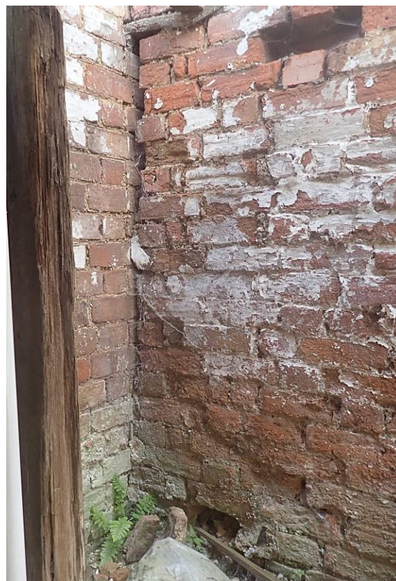
Plate 23 (above). The door from Room 1 in Building 2 to Room 2 with cracking above
