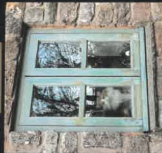
Old flaking timber windows in need of updating and replacing.
