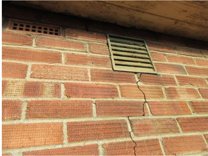
Photograph # 7 (Side – South facing elevation – Crack - high level)
