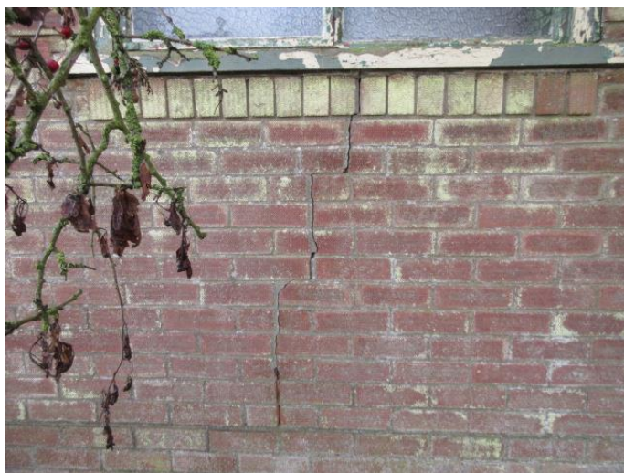
Photograph # 14 (Side – North facing elevation – Adjacent Tree – Crack - mid level - below window)
