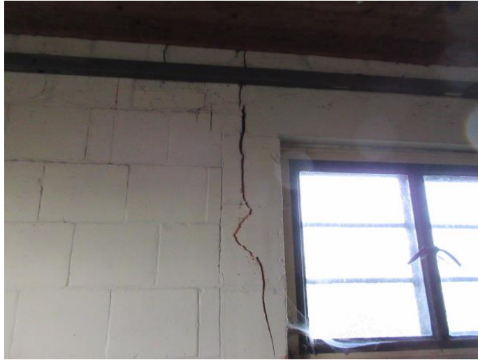
Photograph # 16 (Typical Internal – Side – North facing elevation – Adjacent Tree – Crack - high level - adj window)
