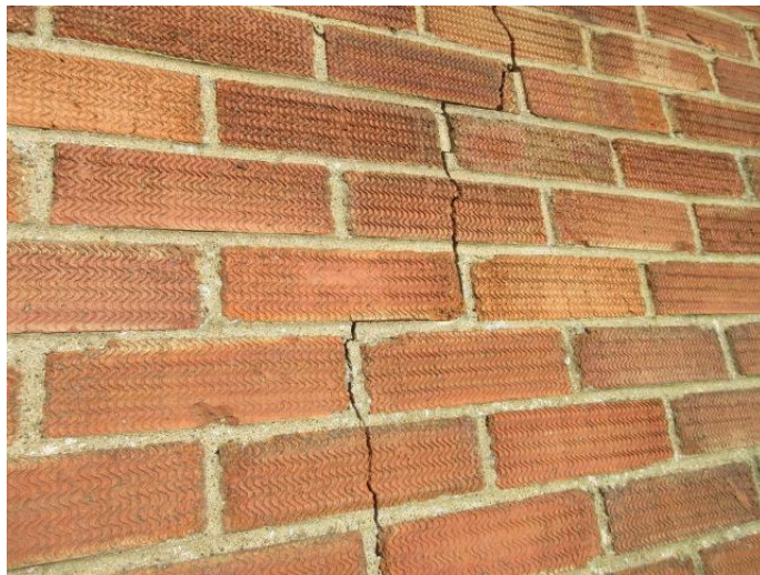
Photograph # 8 (Side – South facing elevation – Crack – mid height level)
