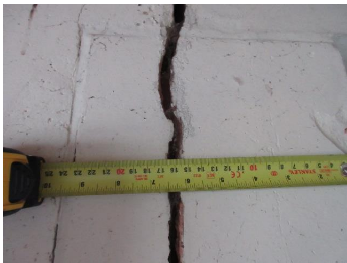
Photograph # 18 (Typical Internal – Side – North facing elevation – Adjacent Tree – Crack - high level - adjacent window)
