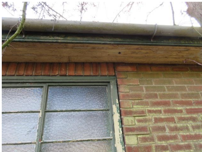
Photograph # 13 (Side – North facing elevation – Adjacent Tree – Crack - high level - above window)
