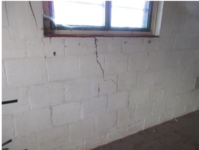
Photograph # 17 (Typical Internal – Side – North facing elevation – Adjacent Tree – Crack - mid level - below window)
