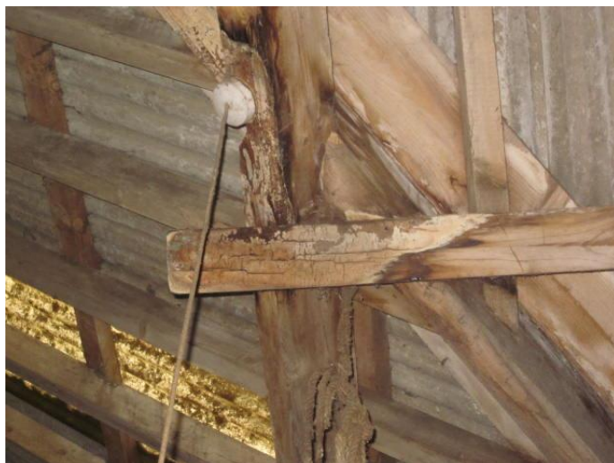
Photograph # 10 Typical Roof – Decay at Valley Intersection.
