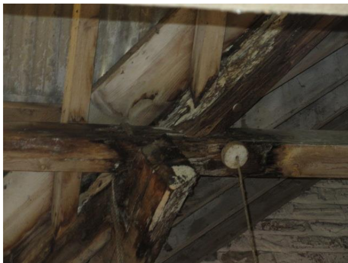
Photograph # 10 (Taken Oct 2021) Typical Roof – Decay at Valley Intersection.
